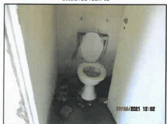
General view of the ablutions. (Note the damage to the cistern)
