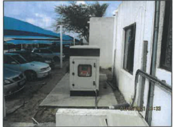
General view of the standby generator
